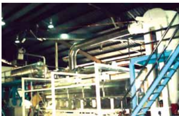
Steam Treatment Plant
