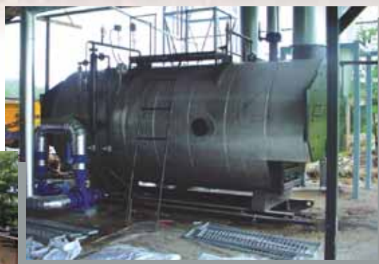
Boiler System for curing leaf
