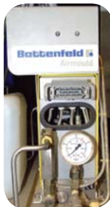
Gas Injection Module
