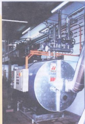
Plate 2 : A modern energy-efficient steam boiler
