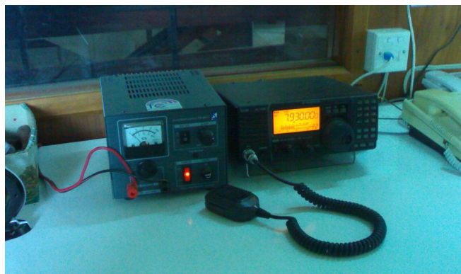
Figure 9.1 Data collection facility for domestic stations
