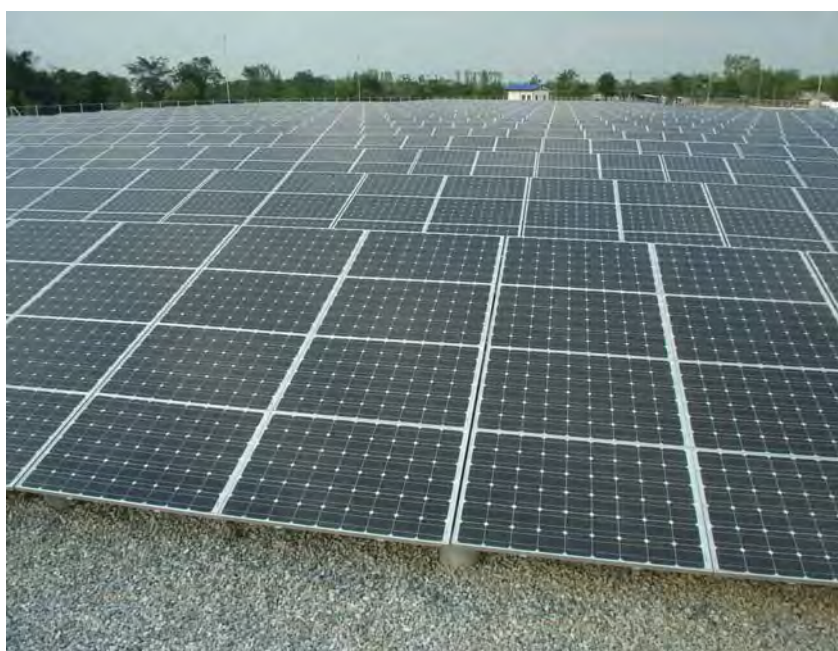
FIGURE 9-8 : A picture of Solar Farm
