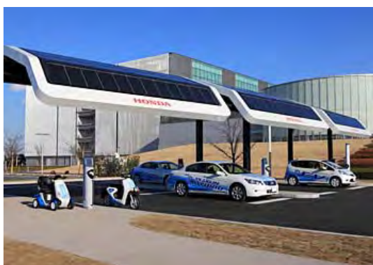
FIGURE 6-17 : Example of charging station ( Saitama City, Japan)
