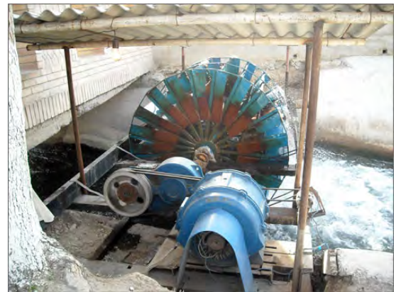
FIGURE 9-18 : Water wheel of small hydroelectric power plants
